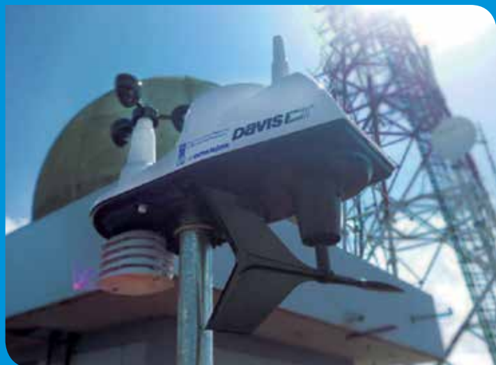
Portable weather station installed in the radar in Pilón which completes meteorological coverage in the south of Granma
